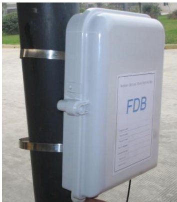
FTTH-005 fiber termination box on the pole
