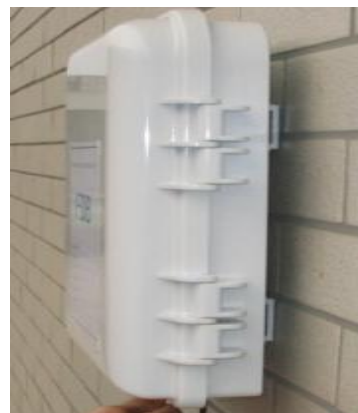
FTTH-005 fiber termination box on the wall
